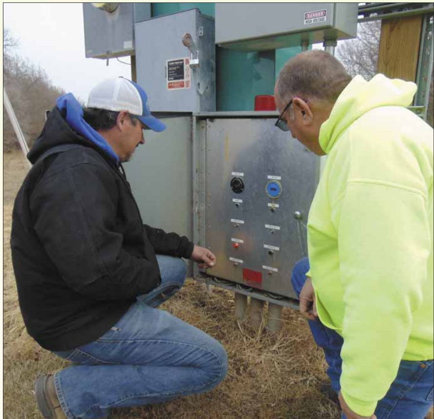
This photo shows city of Wakefield, Kansas Operator Jeff Ochs checking the electrical use hours on the city’s single lift station with KRWA Wastewater Tech Charlie Schwindamann, (on the right). Schwindamann instructed Ochs on the need to check the lift station hours regularly and how to use that information to troubleshoot the lift station and use the same for operational cost evaluations.
